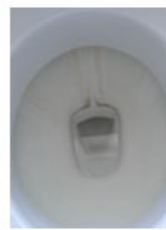
Water scale stains
