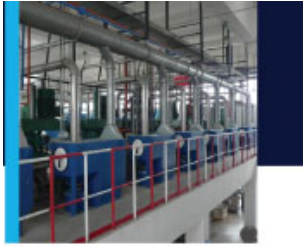
- Sewage Treatment Plants
